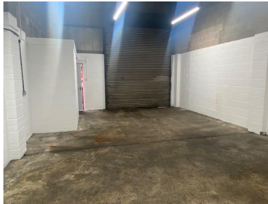
Internal view from rear toward front loading door.
